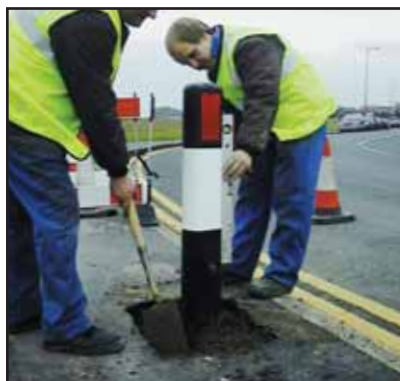
Place gravel to a depth of 100mm into the hole. Bed the Hazardmaster down onto the gravel.
