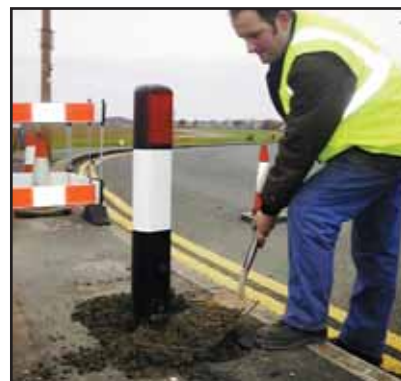
Backfill with concrete and aggregate mix. Ensure the vertical position of the Hazardmaster is maintained during concrete setting period.
